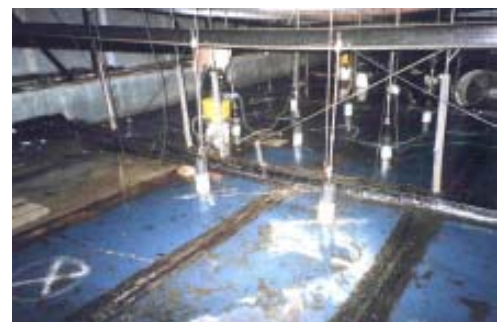
A waterlogged roof void
