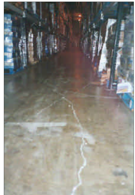
Figure 2 - severe cracks in a cold store floor caused by frostheave
